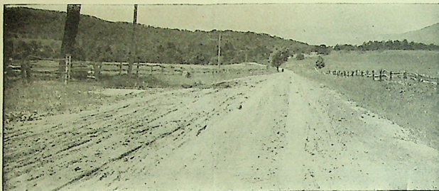
FAILURE OF ROADWAY SURFACE DUE TO POOR FOUNDATIONS
