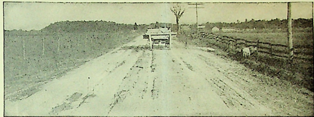
FAILURE OF ROADWAY SURFACE DUE TO POOR FOUNDATIONS
