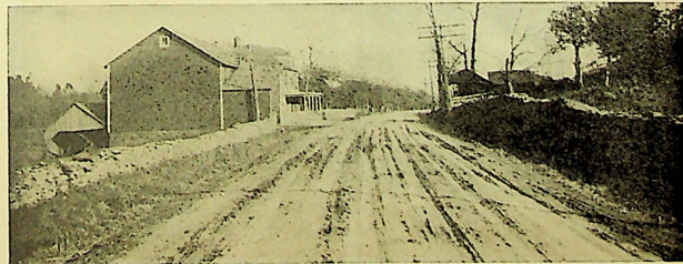
FAILURE OF ROADWAY SURFACE DUE TO POOR FOUNDATIONS
