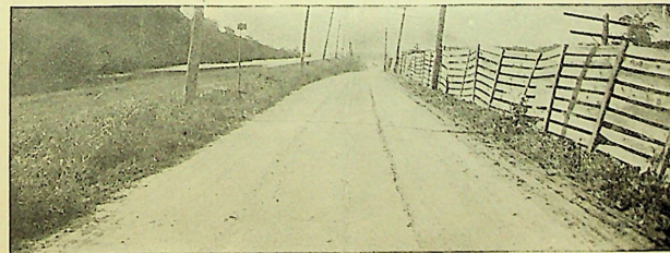
EXAMPLE OF IMPROPER MAINTENANCE
